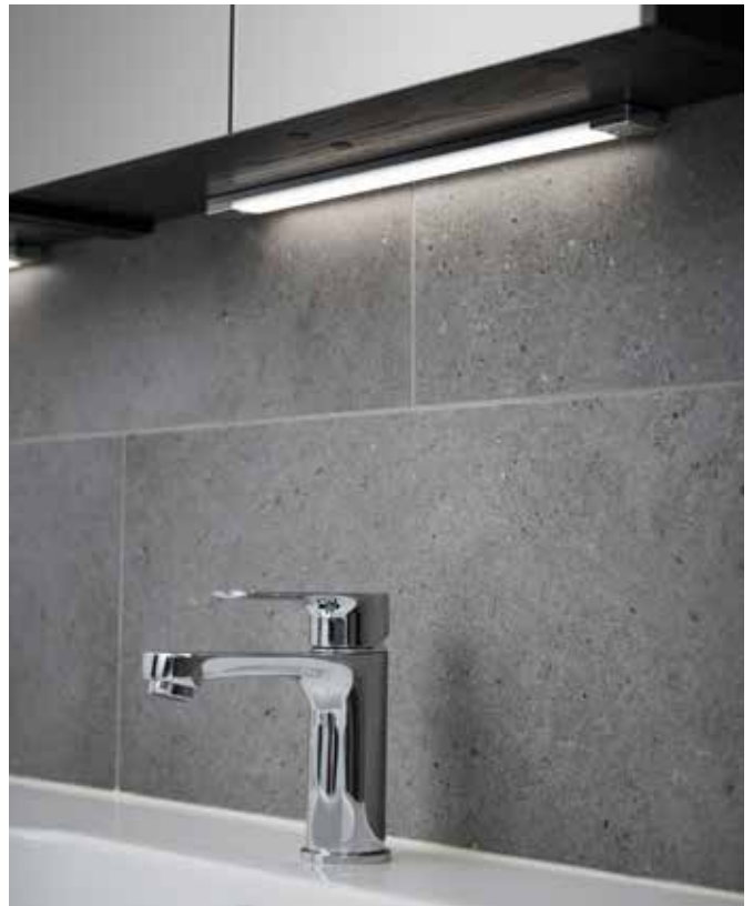
Down light DL2 provides fine lighting above the basin and tap.
